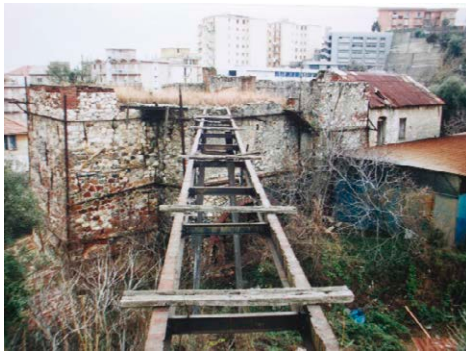
Figure 9 – The track system to transport the quarried stone to the Vallarino kiln.
